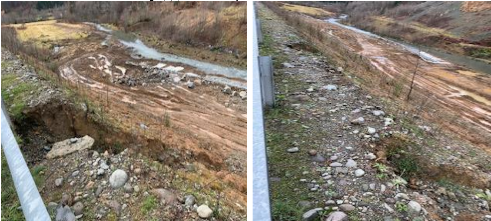
Fig. 1,2,3, 4: Eroded slopes at some sections of the road
