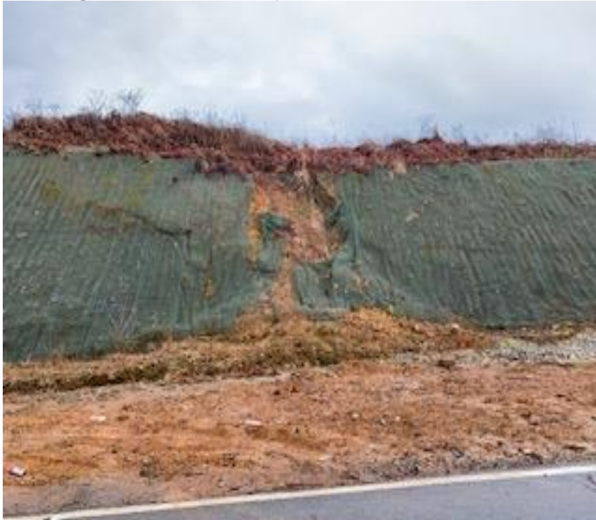
Fig. 8: New eroded slope
